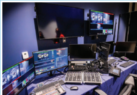
New control room.
