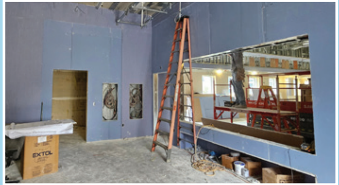
New framing in place for the wall with a large window between the studio and newsroom. Wall in place for new office and new control room.
