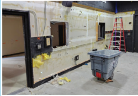
Studio wall being removed to reconfigure into one large window between the studio and newsroom.
